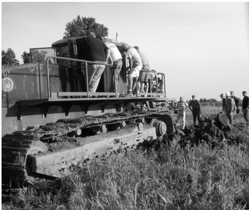
Pictured above is a tile machine which was demonstrated during the field day. Pictured top right, is supervisor, Tim Norris as he discussed tiling installation methods using GPS equipment .
